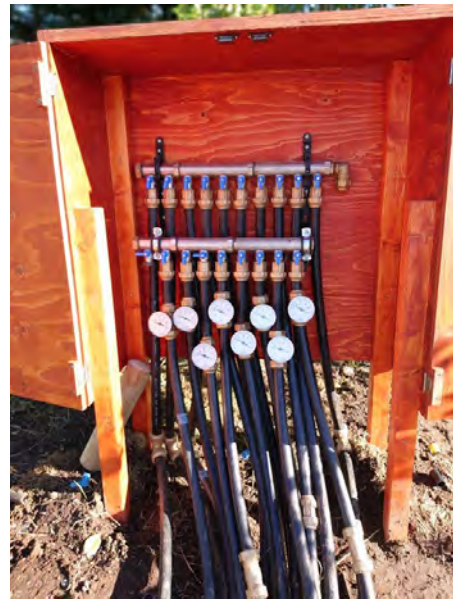
Figure 7: A cabinet built by Arnar Pétursson houses the valve assembly. Pumice was later added at the base.
