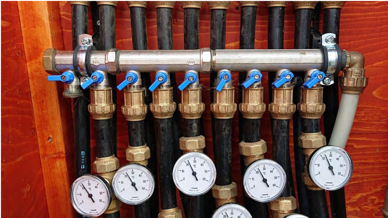
Valve cabinet, visible (top) and infrared (bottom)
