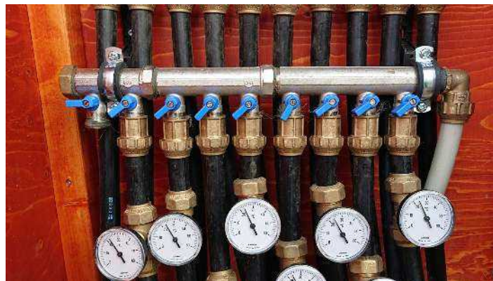
Fig. 1: Valve cabinet for temperature control and monitoring
